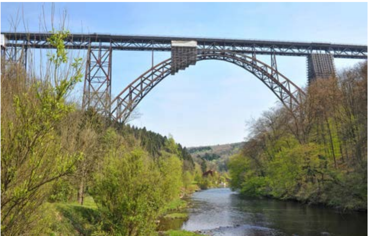
Figure 1: The Müngsten Bridge is the highest steel railway bridge in Germany with a height of 107 m
